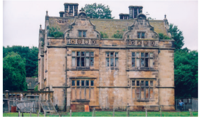
Sockburn Hall in June. The vegetation on the roof has since been attacked with the aid of a cherry picker
