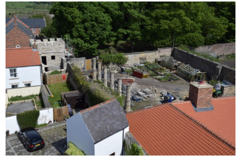
The tower (top left) and west wall seen from the Welcome Tower. The six stone columns are what remains of a 17th-century hay barn inside the Castle wall.
