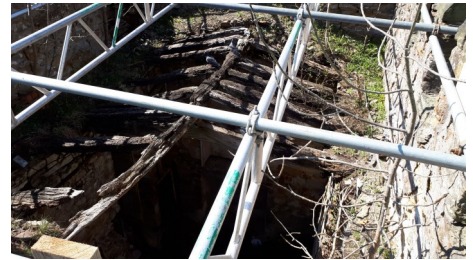
The decayed roof showing the close-set big rafters; the craftsman who reconstructed the roof said ‘you could stand an elephant on that.’
