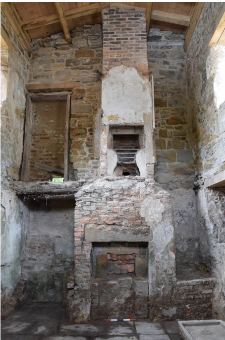
The east wall with the restored roof in place. The chimney is a later addition that hides older fireplaces
