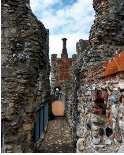
View along the wall-walk at Framlingham Castle to Tower 6 with an inserted Tudor chimney
