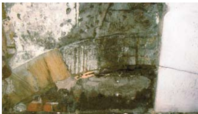
The upper order of the tower arch. This walling is now hidden behind a false wall at gallery level.
